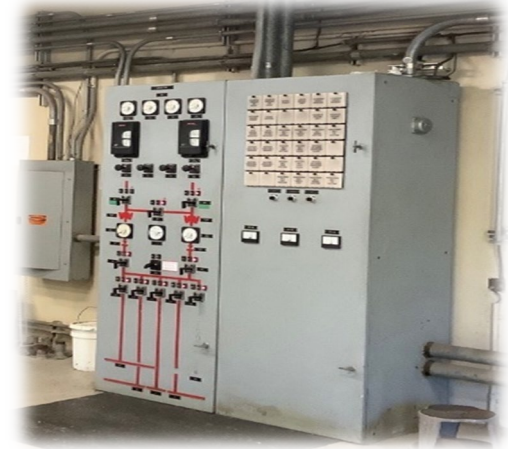
Main Breaker Panel
